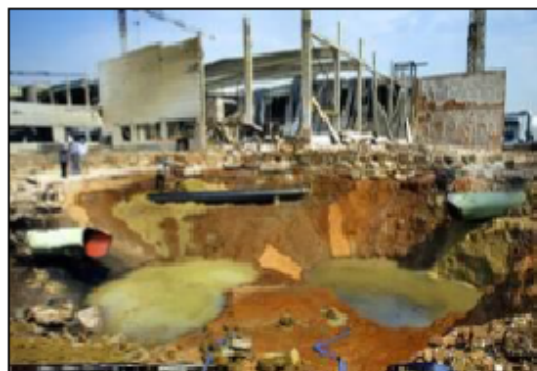
Figure. 2.Explosion happened due to pipe leaking [3].
