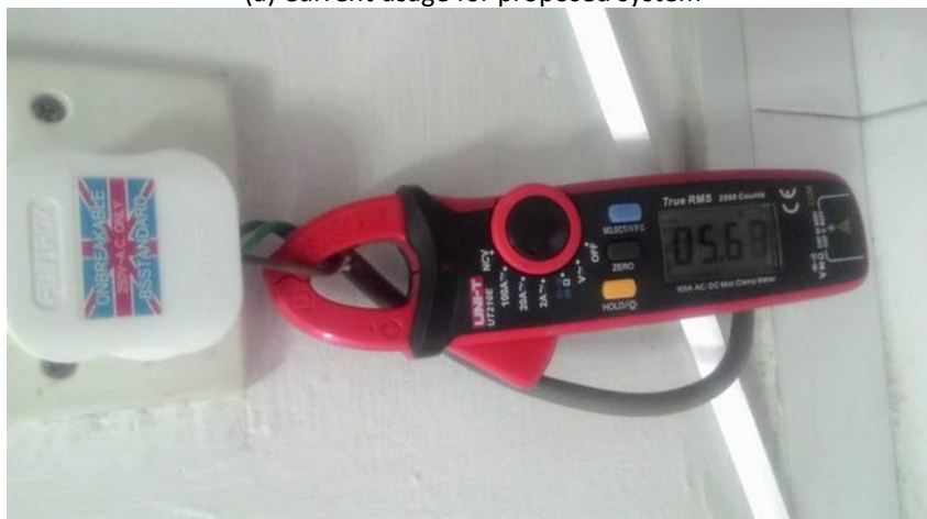
(b) Current usage for 1 horsepower conventional air-conditioning
