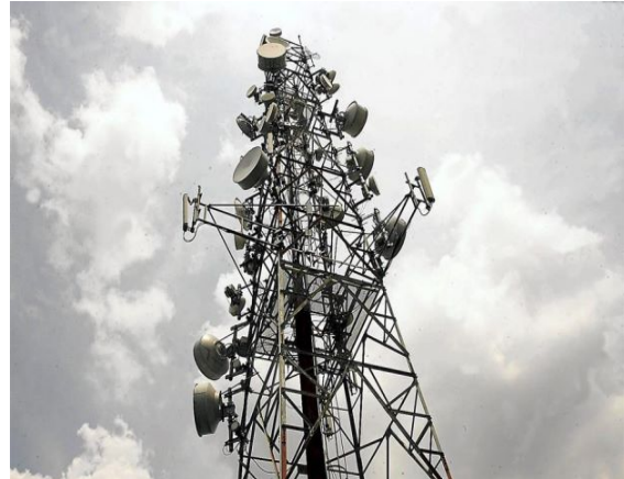
Fig. 1: Example of base transceiver station tower
