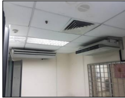
Figure 4. Comfort cooling system in Politeknik Muadzam Shah data centre
