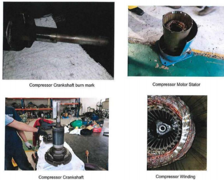
Fig. 1. Semi Hermetic Compressor Mechanical Failures under Study
