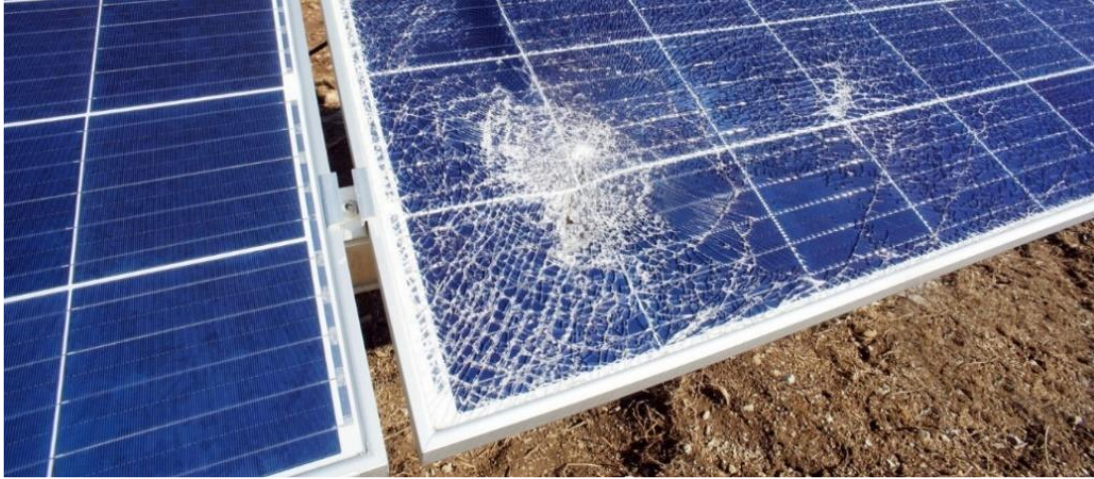
Fig. 5. Cracks on solar panel [50]
