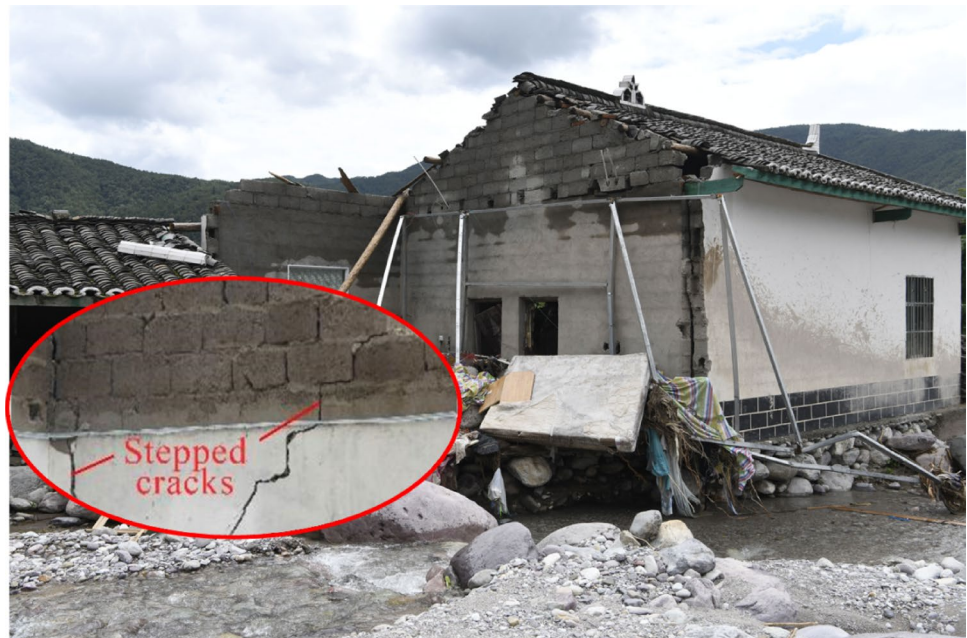
Fig. 2 Damage to a masonry wall resulting from flash floods in Wenchuan, China, reproduced with permission from [6]
