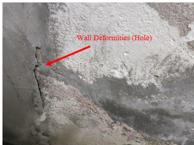
Figure 17 Uneven wall picture
